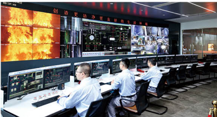
Central Control Room in Xi'an Gaoling WtE Plant
